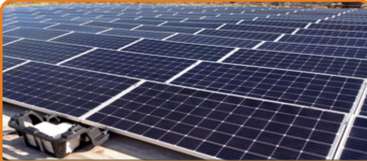
Photovoltaic panels at Honokanai'a base camp.
